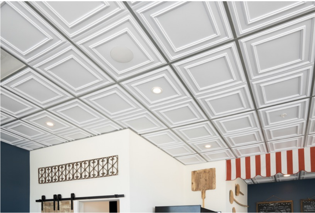
In the re-designed ceiling, all lights and sprinklers are properly placed for balanced appearance, and an air grate equalizes air pressure above and below the ceiling.
