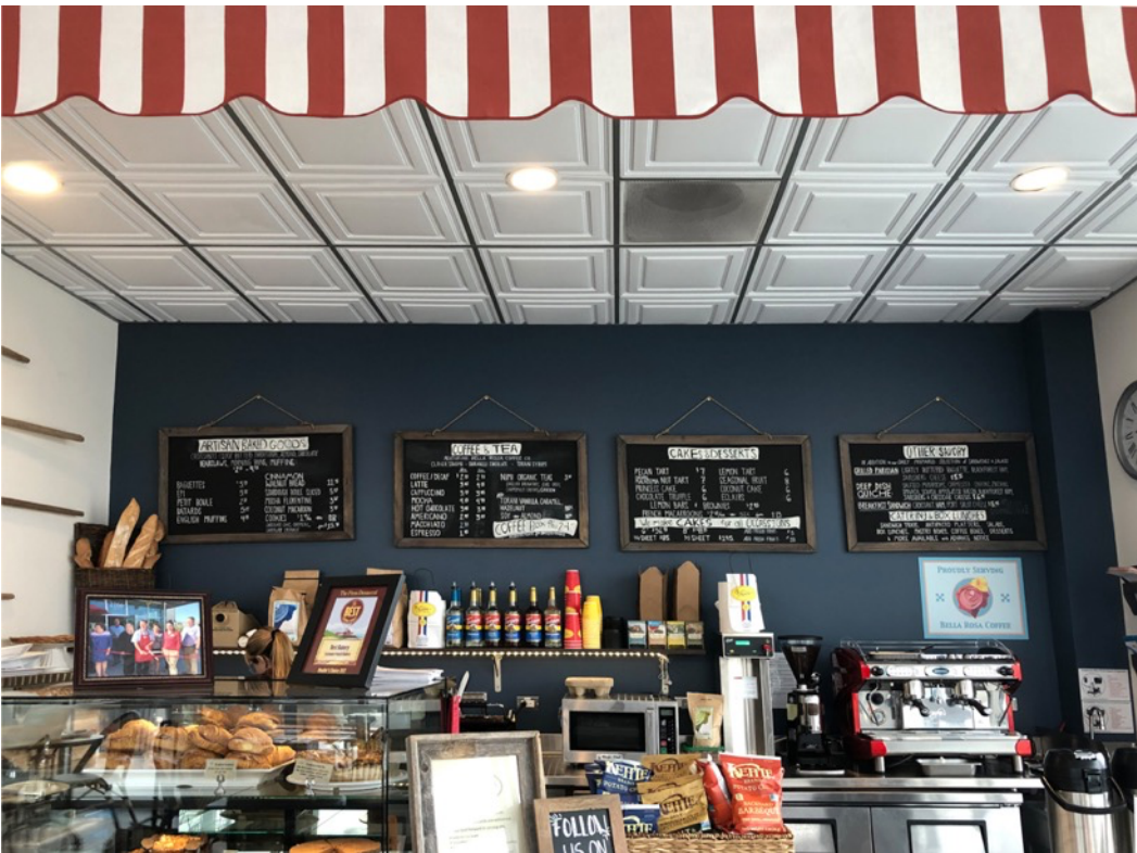
The original installation of the ceiling included mistakes, such as recessed lights placed in the center of a 2x4 tile, in the divide between the two squares. They were relocated during the re-design that solved the wind uplift problems.
